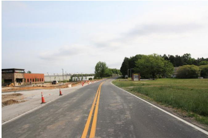
STREET – Facing northeast along E. Butler Road Site is undeveloped property to the left New commercial under construction adjacent to site can be seen in distance on the left
