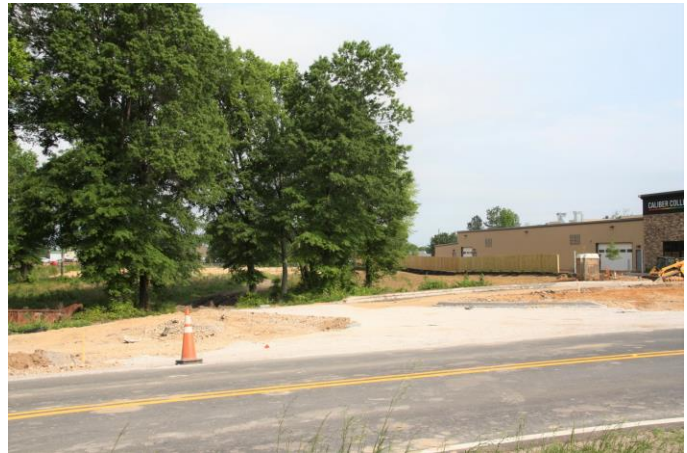
SITE – East edge of site Facing northwest from Butler Road Site is wooded property on the left New commercial building under construction can be seen on the right
